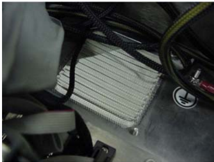
Figure 67: Blow Out Filters
